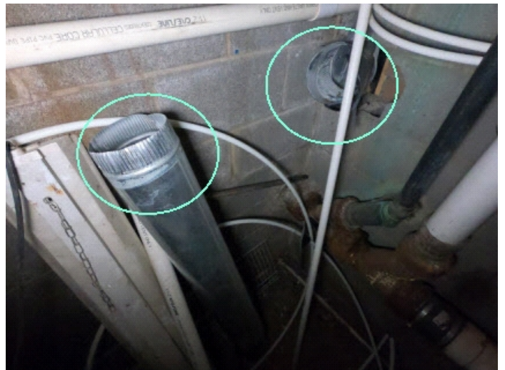
Furnace ductwork loose and not connected.
