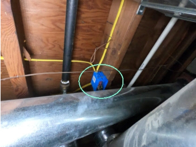
Numerous areas have sloppy wiring or require cover plates.
