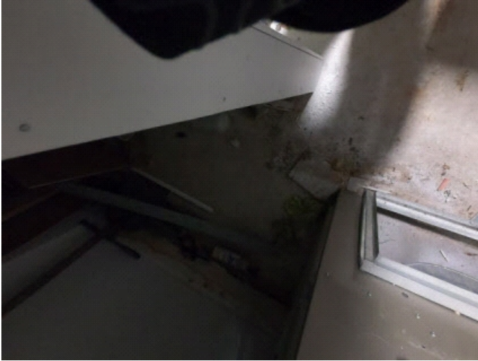
HVAC ductwork may need cleaning and filter.
