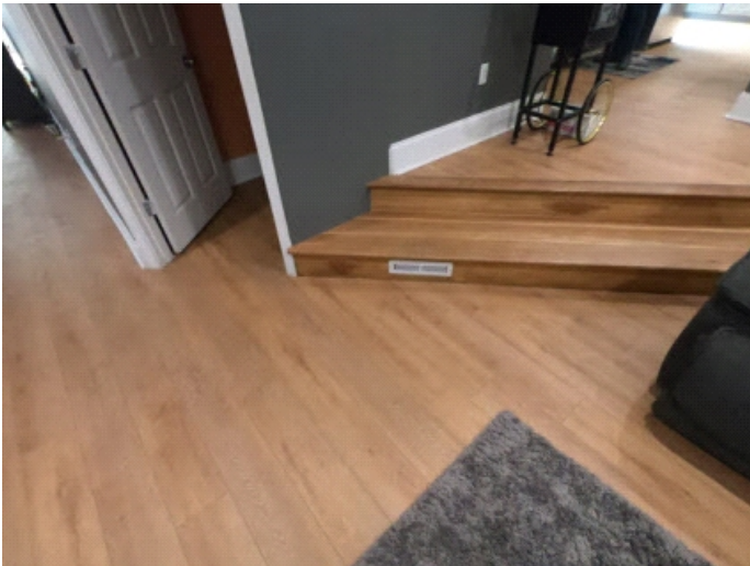
No access under steps or crawlspaces or under slab's.
