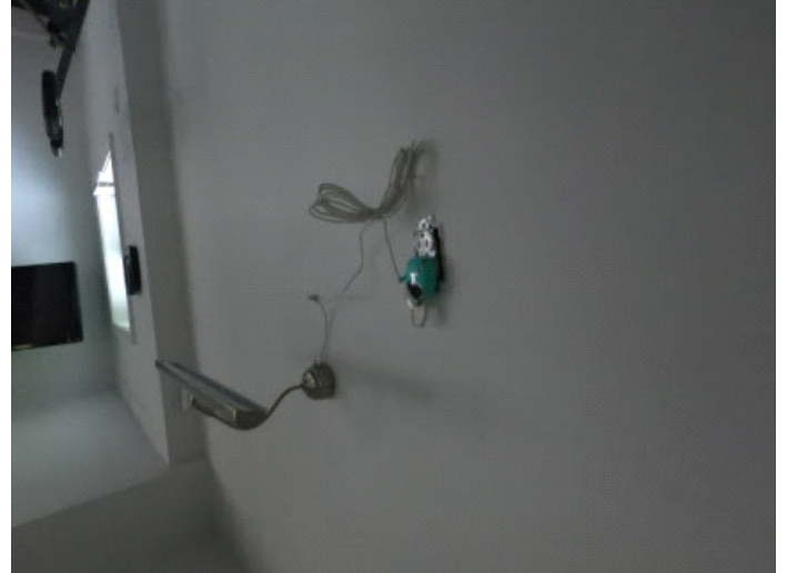
Some electrical outlets need cover plates
