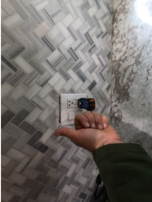
GFI's properly function.
