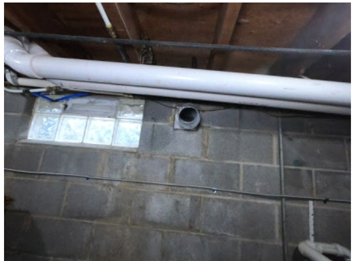
Vent not connected. Caulk and insulation around perimeter.
