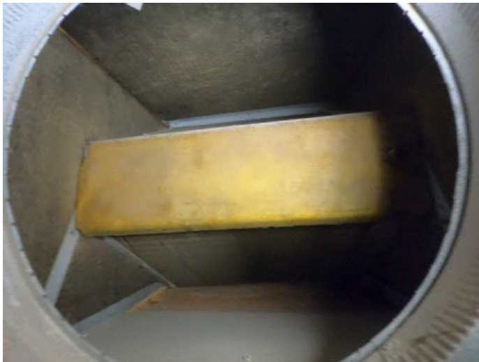
The air handler in attic nonfunctional and appears to be abandoned. Recommend removing.
