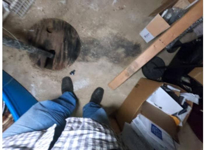
Recommend sub pump cover that is one or percent sealed and not wood. Should periodically check battery backup once installed.
