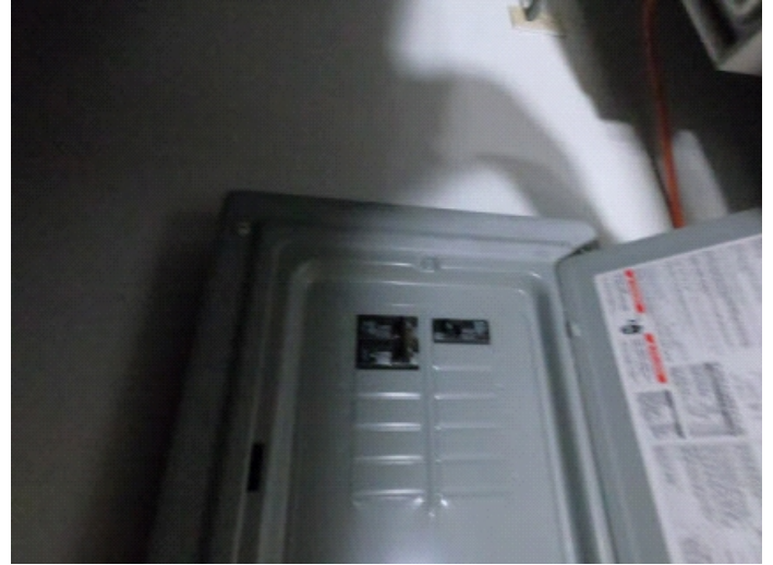
Some electrical wiring could be in conduit.
