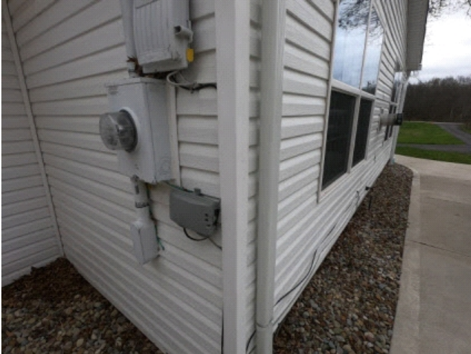
The main electrical meter.
