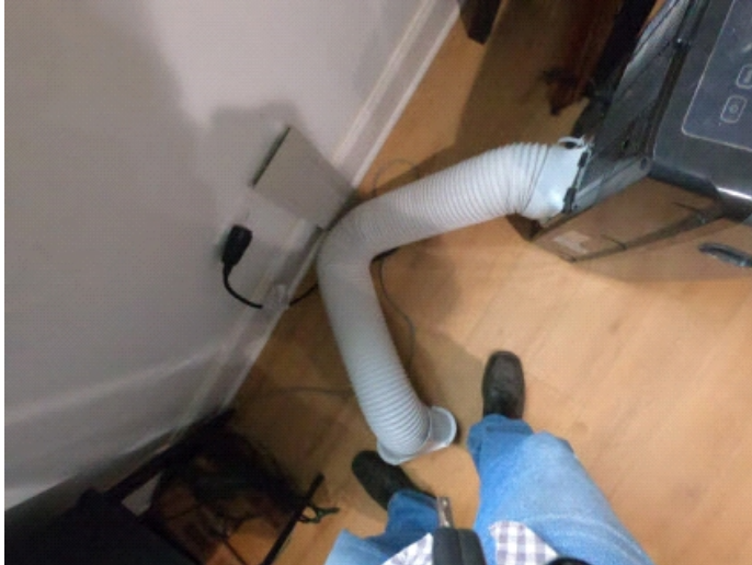
Garage second floor may need supplemental AC.
