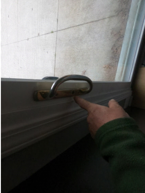
Sliding door lock needs adjustment.
