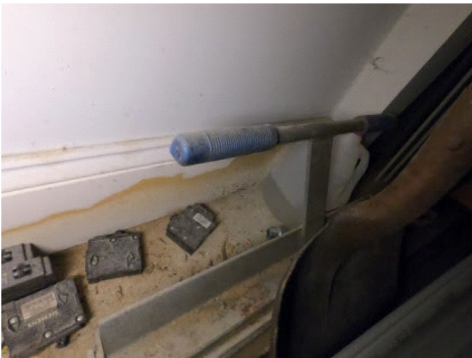
Some old stains from exterior moisture intrusion. This appeared to be an old leak or other and was dry at time of inspection.
