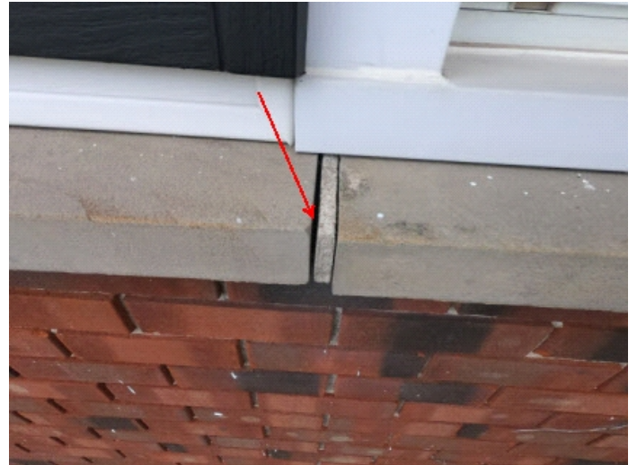
Some maintenance tuck pointing recommend.
