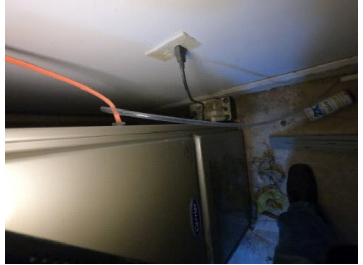
Discharge pump not connected.
