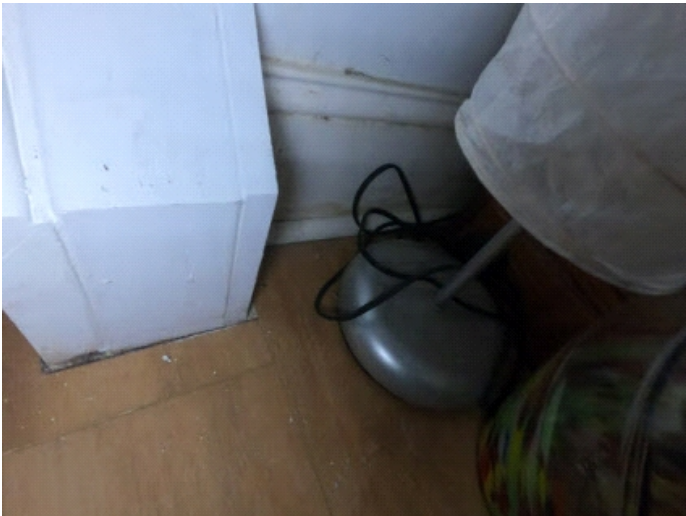
Some old water stains and basement walls. These were dry at time of inspection.
