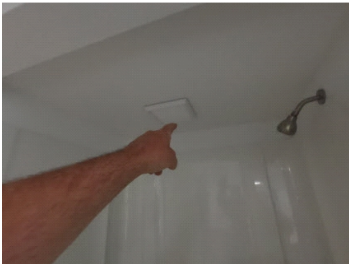
Some light bulbs are burned out or nonfunctional.
