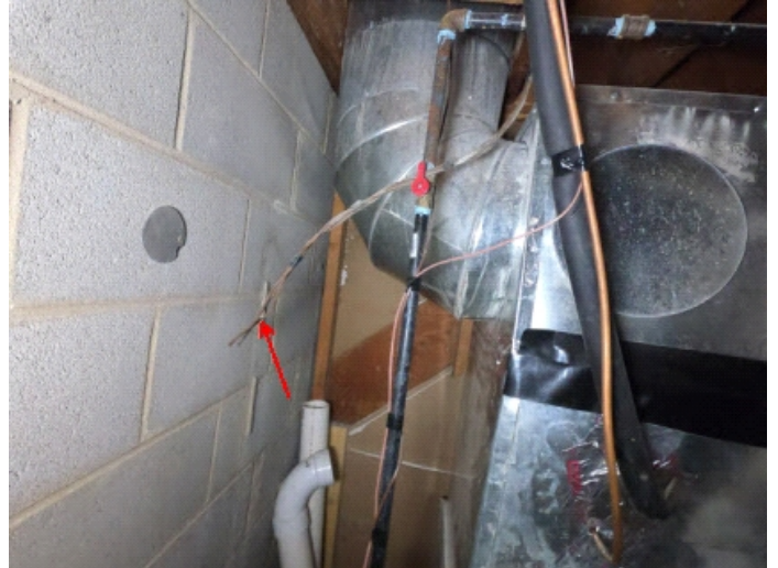
Unknown low-voltage. low voltage, phone, cable and other subsystems not evaluated.
