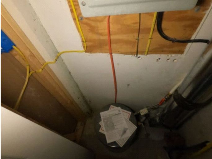
Electrical should be in conduit.
