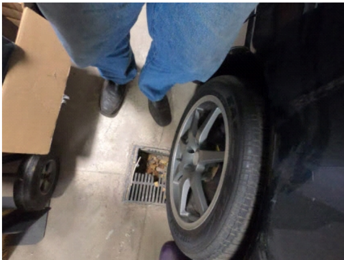
Need new drain cover.
