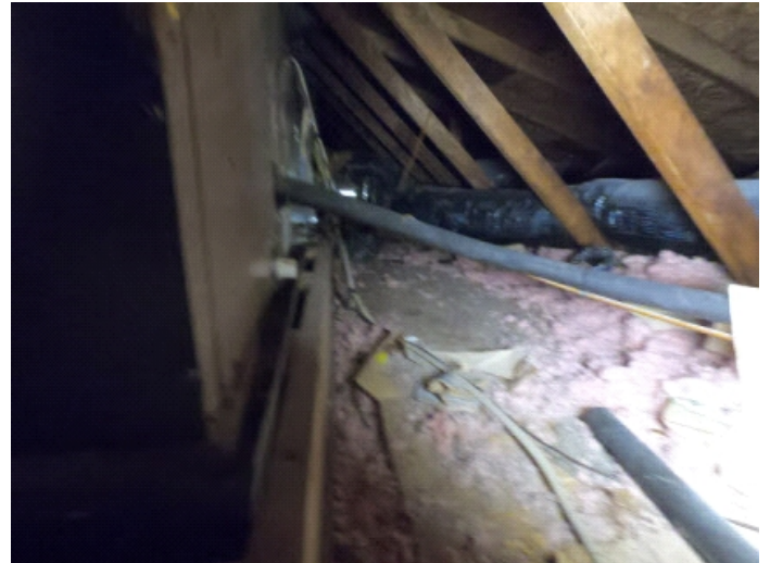
Could improve insulation in the upper attic. Sloppy electrical an upper attic. Some mildew or mold in sheeting ( isolated).
