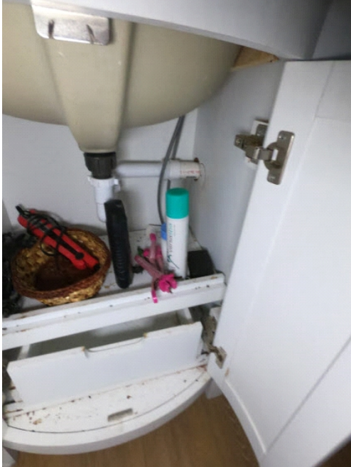
Drain needs adjustment.
