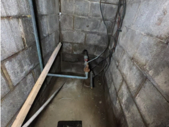
Main water line with pressure reducer.
