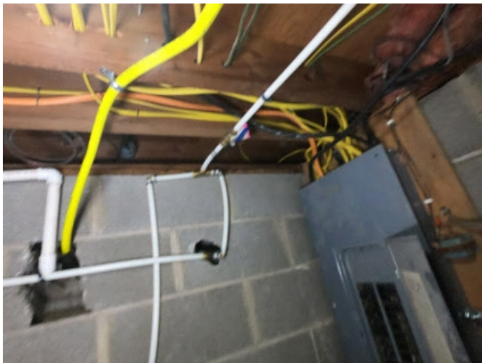
Plastic, PEX and copper domestic plumbing.
