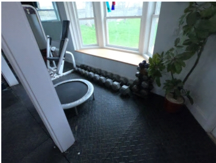
Windows may need cleaning to check to make sure if seals are good.
