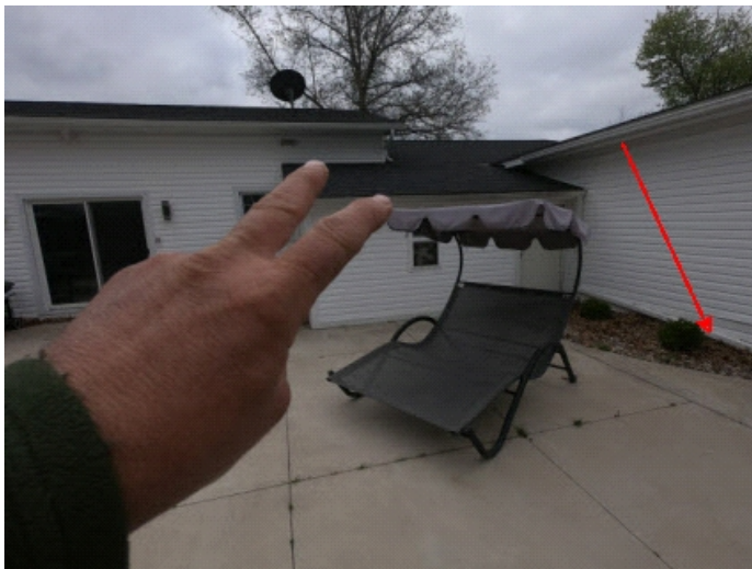
Foundation grading is a bit flat. We were informed that this area has a recent trench drain installation.
