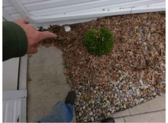
Horizontal downspout installation. Sometimes these leak.
