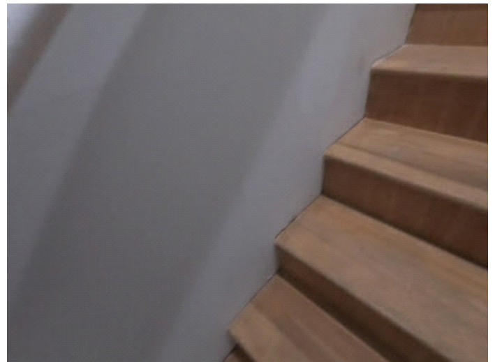
Drywall a bit sloppy.
