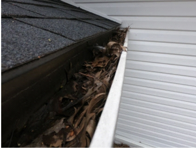
Gutters and downspouts need maintenance, cleaning and or adjustments.
