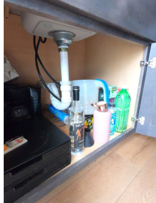
No leaks under most sinks.
