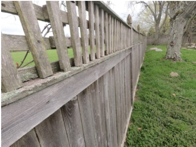
Old fence with wear and tear.
