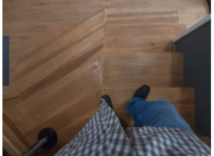
No handrails for steps.
