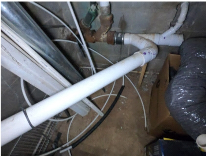
Most drains were PVC.
