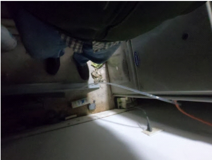
Furnace discharge drain is not connected.
