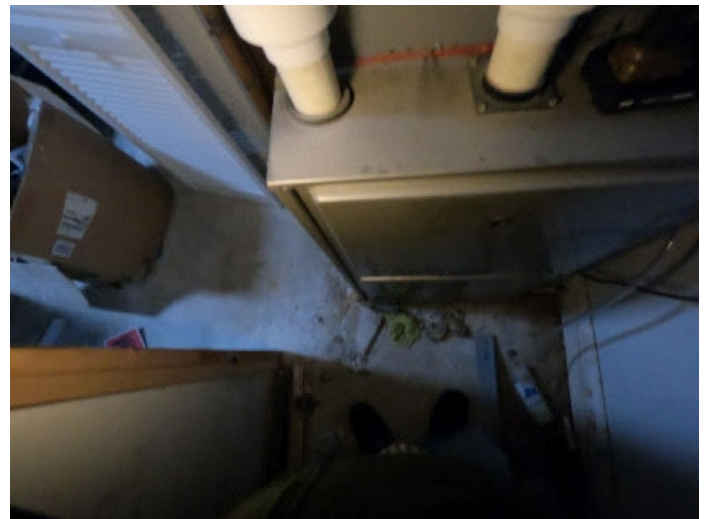
No air-conditioning for garage, workout room or finished garage rooms.
