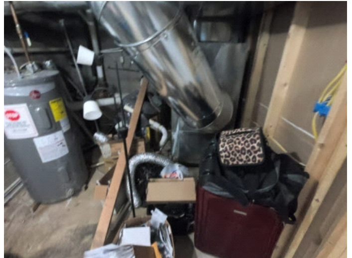
Sylvester things close to HVAC units. No drain pans for electric water heaters.
