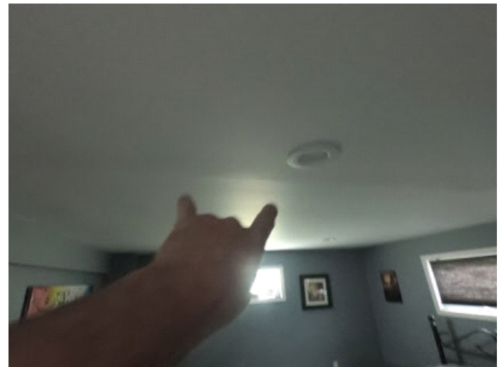
Bed rooms do not have cold air returns. Some people will cut bottoms of doors to bring return air to cold air returns. Living room has cold air returns.
