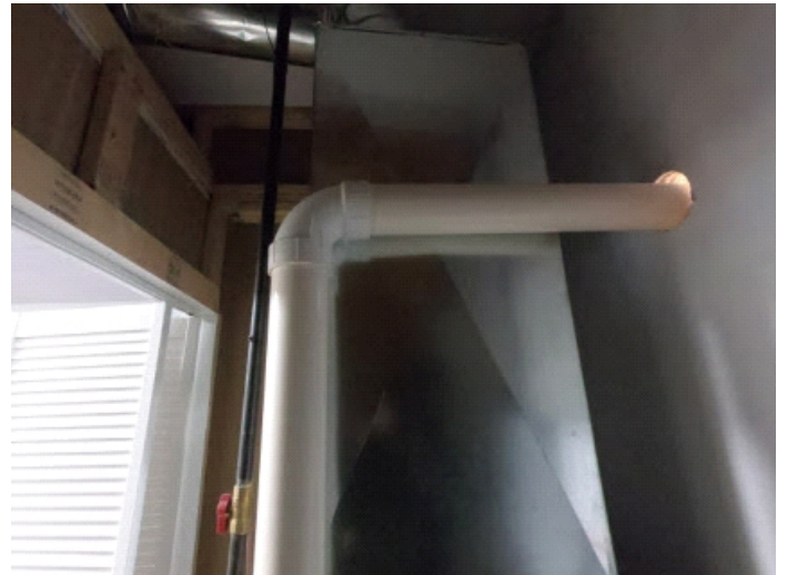
Furnace flue needs to be sealed and waterproofed to the exterior.
