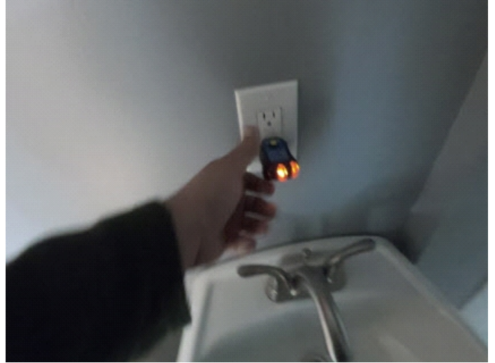
Outlets properly function.
