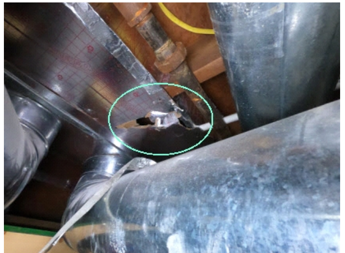
Cold air returns in basement need to be sealed to minimize negative pressure.
