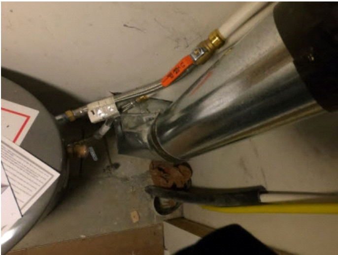
Small electric hot water heater located in garage. No floor drain in this utility closet.
