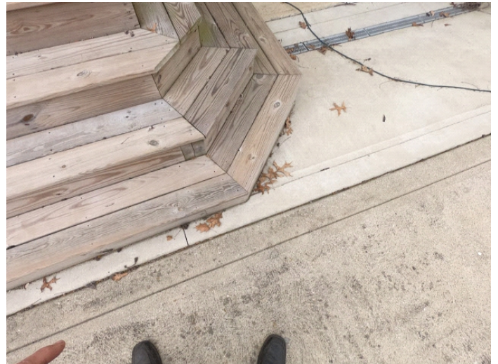
Older wood steps. No hand rail. Keep trench drain clean and operational. It was not raining at the time of inspection.
