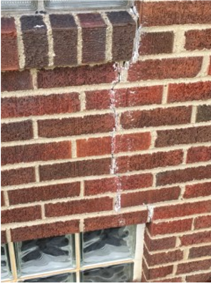
Vertical crack at the rear wall beneath the glass block window
