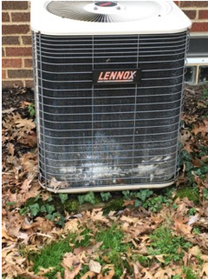
1998 Lennox air conditioner
