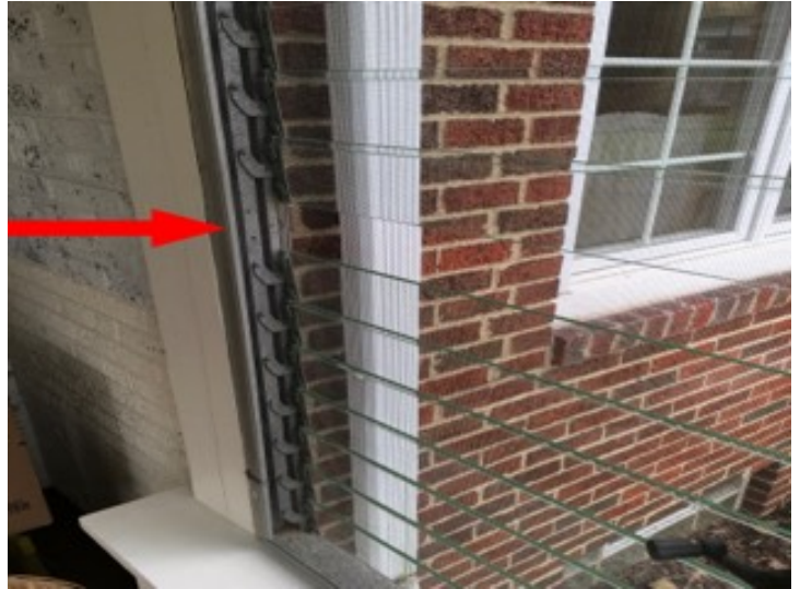
Missing pane and opening mechanism.
