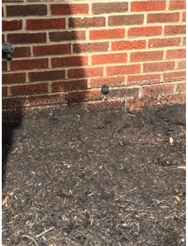
The front gutter is overflowing and splashing debris on the wall and moisture is penetrating the front bay window.
