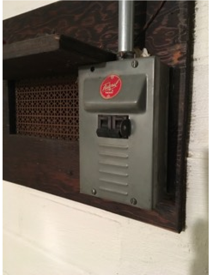
Recommend replacing the Federal Pacific breaker panel in the furnace room. Safety issue.
