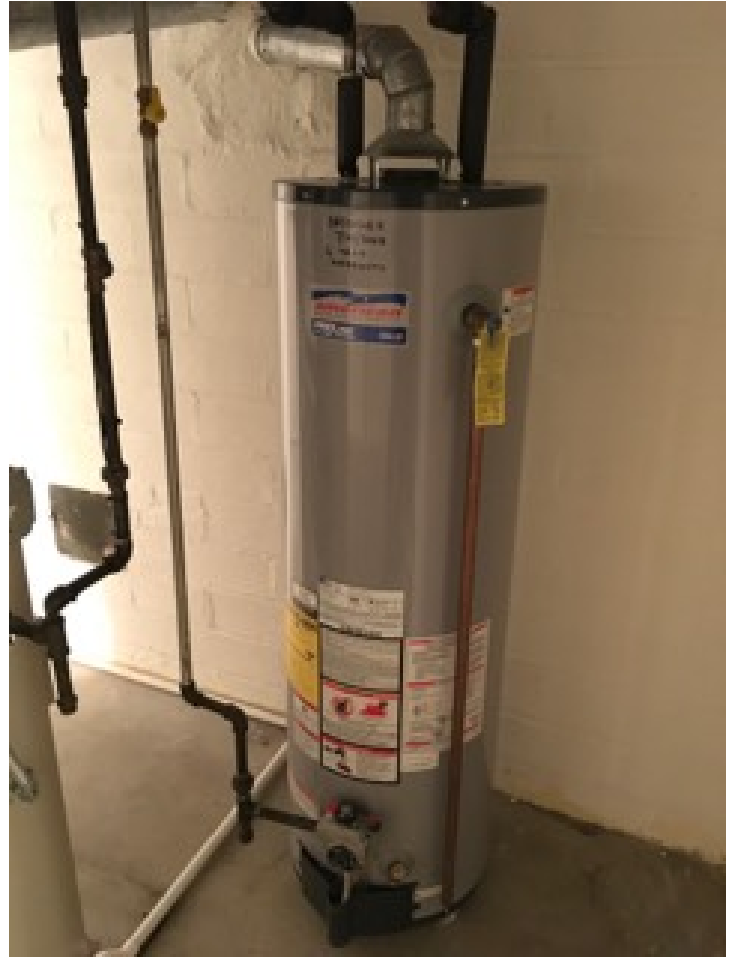
2008 American hot water tank
