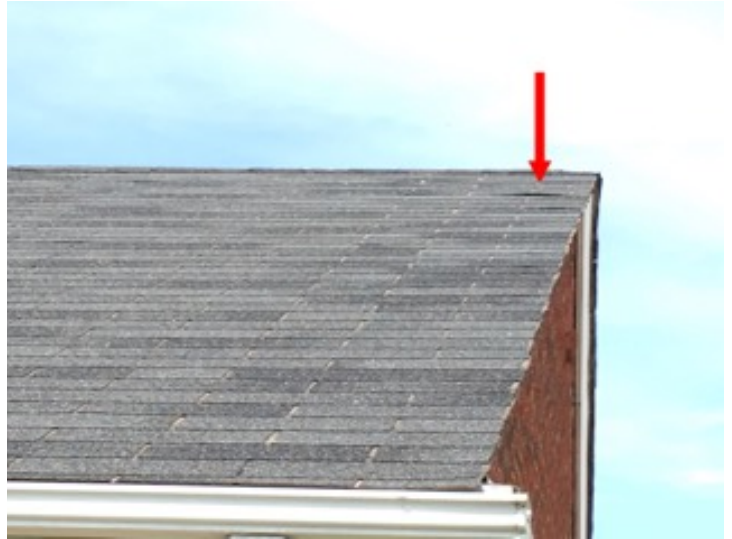
Minor cupping at the front roof
