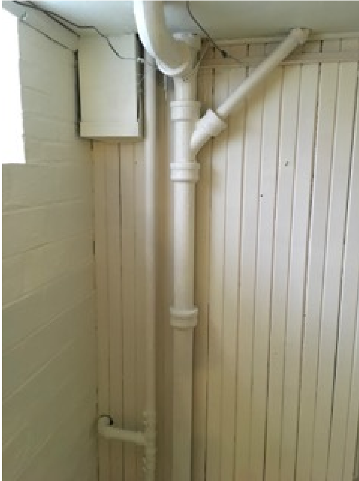
Cast iron drain pipes
