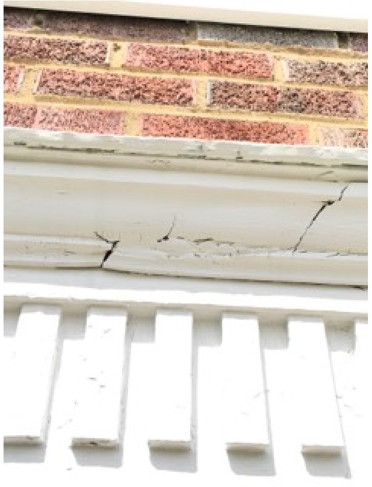
Trim damage above the garage door
