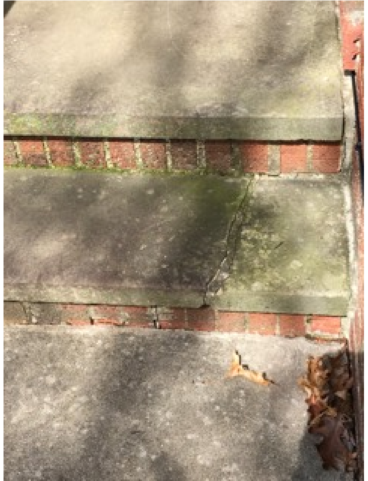
Cracked stone at the side entrance
