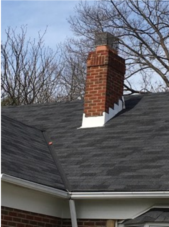
Front chimney has loose mortar joints and flaking
