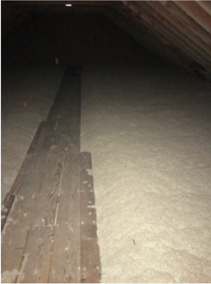
A blanket of insulation in the attic
