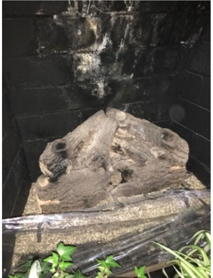
The gas logs were not operated at the inspection. The gas valve was turned off in the basement.
