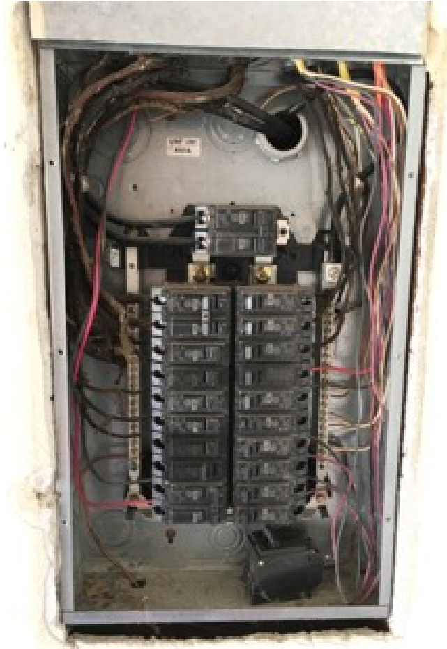
100 amp main breaker panel is properly installed and appears to be grounded
