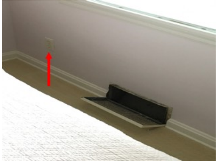
Loose heat duct cover and ungrounded three prong outlet at the north wall of the northeast bedroom
